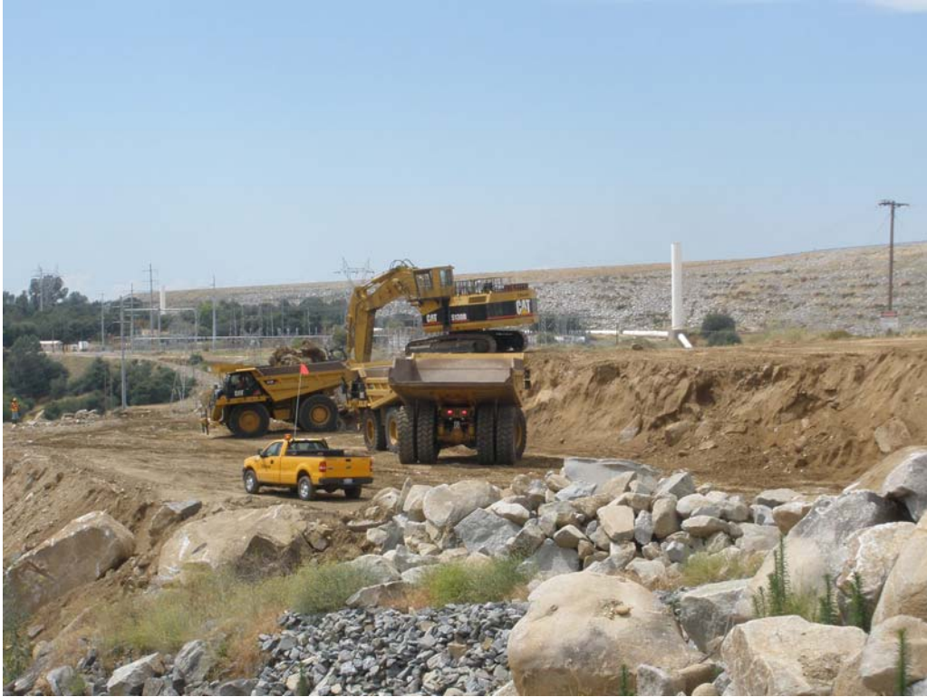
View of the 5130 excavator and 777 haul trucks at about station 33+00 of the spillway excavation
