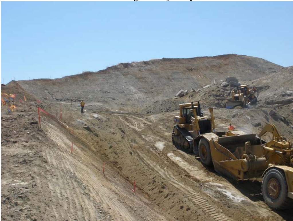
Looking east in spillway at about station 13+00 (D10 push CAT pushing 651 scraper)
