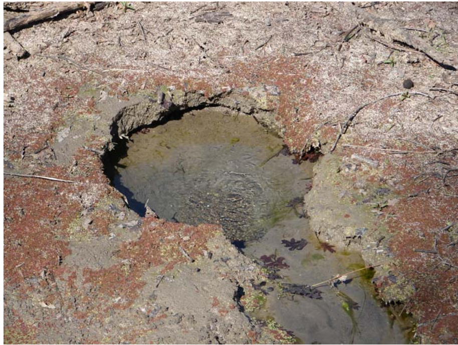
Photograph No. 2: Close-up of Boil in Pritchard Lake Intake Canal (03-04-08)
